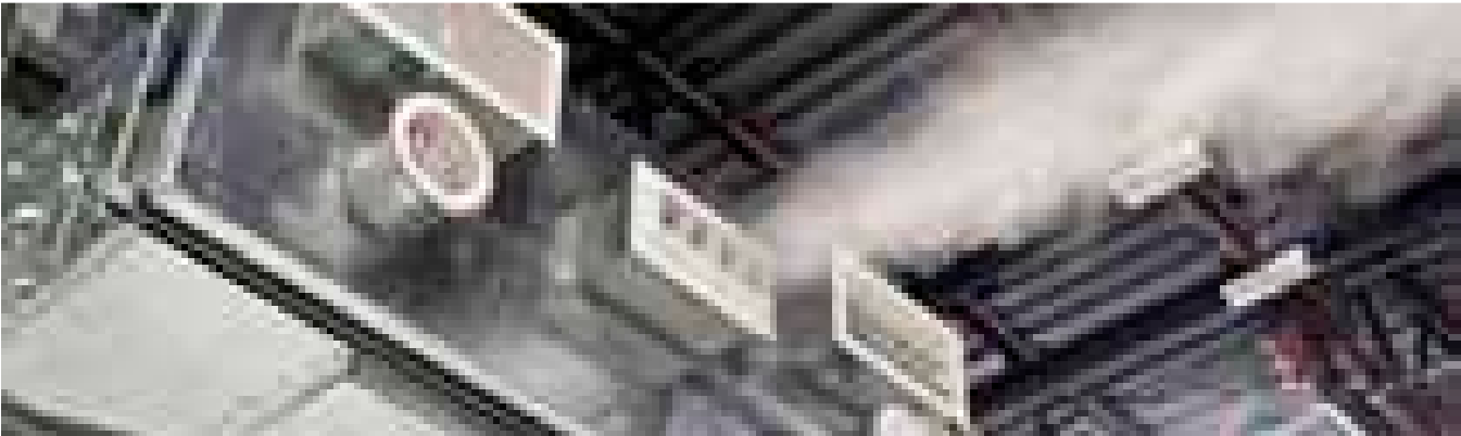
Our Air Moving product divisions rely heavily on our Air Moving Test Areas, Nozzle Diffuser Demonstration Area (shown), High Bay Diffuser Area, Psychrometric Chamber and Fan Coil Test Chamber for testing products large and small
